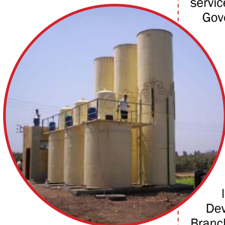
Wastewater treatment facilities will be locally constructed and managed at the rural village level
