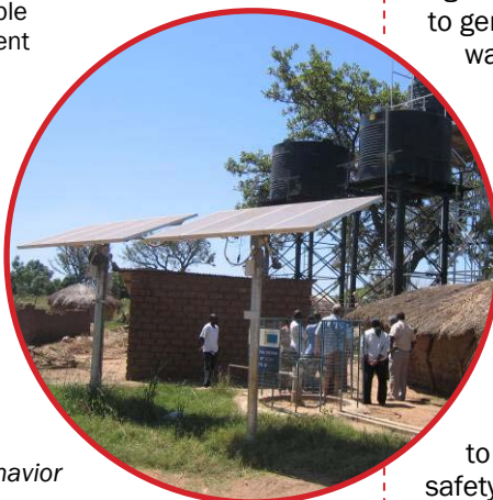
WADA constructed high volume solar-powered water supply provides populations returning from prolonged conflict with water for drinking and agriculture
